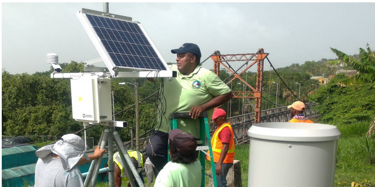
TaiwanICDF employed Taiwan's experience in disaster prevention to help allied countries improve their monitoring and set up an early warning mechanism. Capacity-building, education, and training were also provided to improve their technical capacity for disaster response. (Pictured is the Belize Urban Resilience and Disaster Prevention Project)
