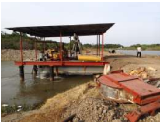
Photo 5. Pumping station in Punta Chame.
