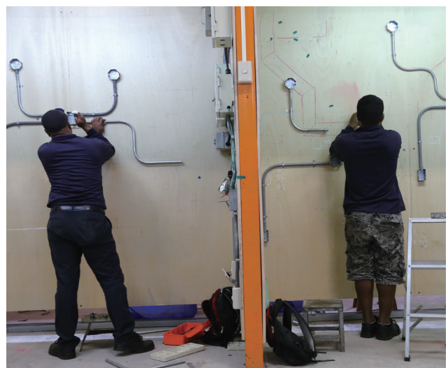
One of the TaiwanICDF's educational reforms is transforming from an "elite-type framework" to "Education for All," an initiative advocated by the United Nations. (Photo shows youths working on electric and plumbing as part of the Taichung-Changhua-Nantou Regional Branch Vocational Training Project for Youth in the Pacific. )
